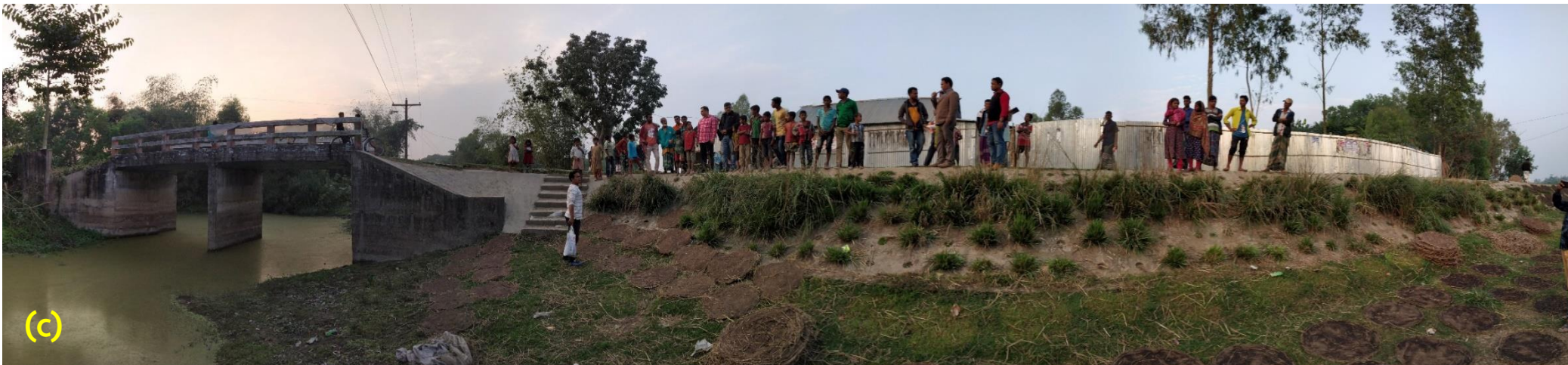
(a) VGT applied to a bridge approach road; (b) Side slope protection of a submersible road (which remains inundated every year for 4-6 months during monsoon) located in a haor area; (c) Steep slope protection using vetiver grass planted in hollow CC block (1000mm × 1000 mm × 100 mm with 75mm dia hole at the centre) holes where growth is hindered due to poor maintenance (Islam, 2020a).
