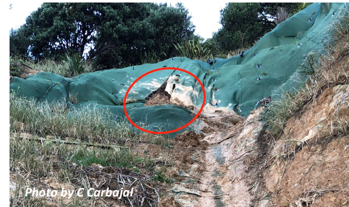
Failure of soil nails and geotextile
